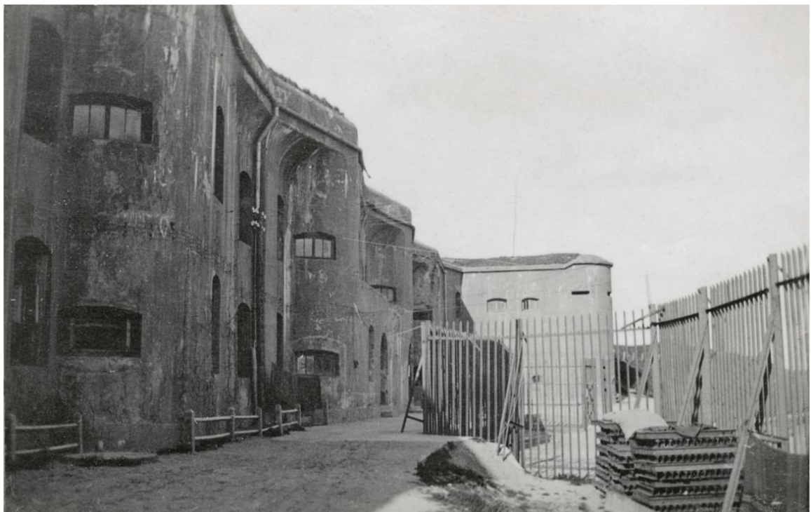
Courtyard of the barracks of the Ninth Fort of Kaunas Fortress with a semi-caponier in the background, 1915-1916. © Bayerisches Hauptstaatsarchiv
